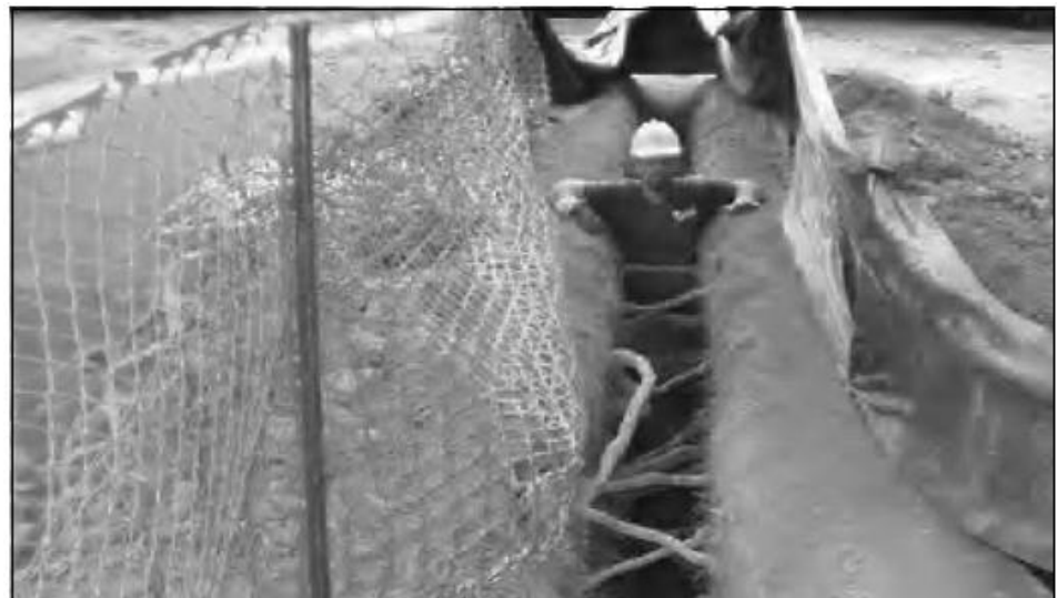
Air spades (radial trenching) can be used to break compaction under existing trees. Exposed roots must be protected from desiccation.
