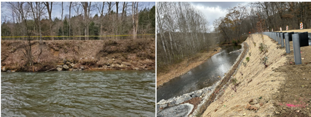
On the left, is a before picture of the slide and, on the right, is a progress picture of construction at Fisherman's Cove
